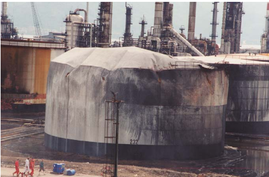
Fig. 1 : Deformation of cylindrical tank with fixed roof after the 17 August 1999 Marmara Earthquake at the Tupras Refinery.
