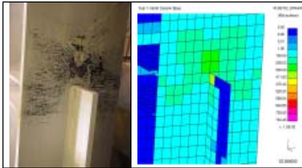
Figure 11 Column Stiffener Plate Yielding
